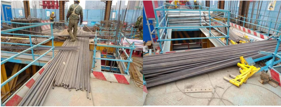
Figure 18. The situation of stacking steel bars at the edge of the opening
